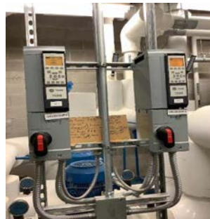
Chilled Water Pump Controls
