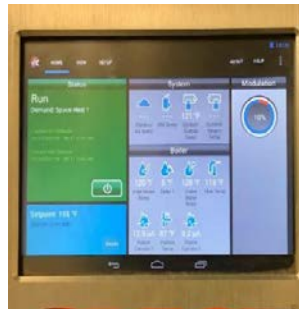
Boiler Display Screen
