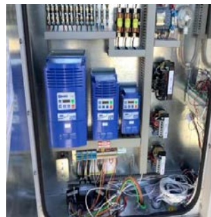
DOAS-2 VFD Controls
