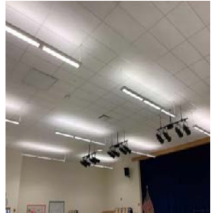
Cafeteria Pendent Mounted Lighting Fixtures
