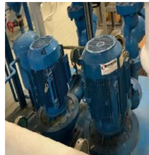
Heating Hot Water Pumps
