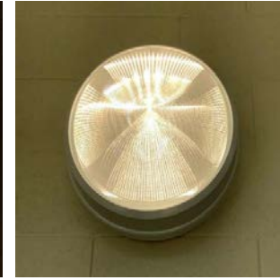
Stairwell Wall Mounted Fixture
