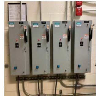
DHW Circulation Pump Controls
