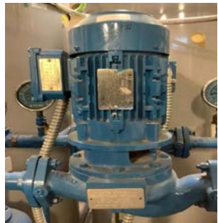
DHW Circulation Pump 1B
