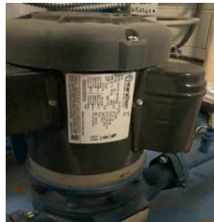
DHW Circulation Pump 2A
