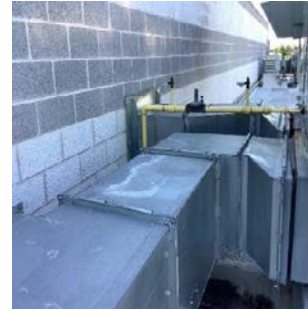
RTU-3 Uninsulated Ductwork
