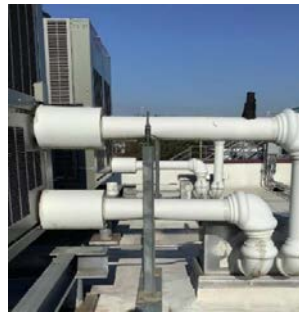
Insulated Chilled Water Lines
