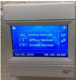
Automated Lighting Control System
