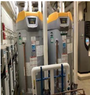
DHW Storage Tank Water Heaters
